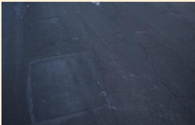
Cracking and covered pot holes
